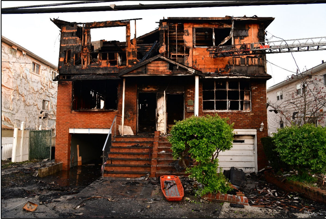
Figure 9. Aftermath of incident at 10826 and 10824 Avenue N, Brooklyn, Box 3-3 2075 (front elevation).
