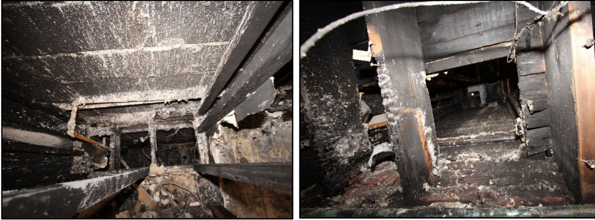
Figure 46. View of vertical shaft on the first floor looking down (left); view of vertical shaft from the basement level looking up (right).
