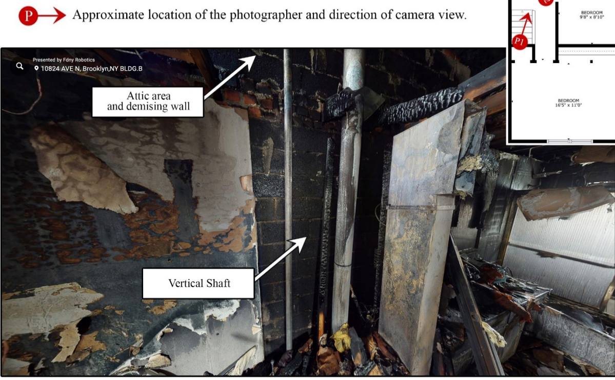
Figure 18. View of the second-floor hallway and iron railing (top); view of the second-floor vertical shaft for flue pipe and HVAC vent (bottom).
