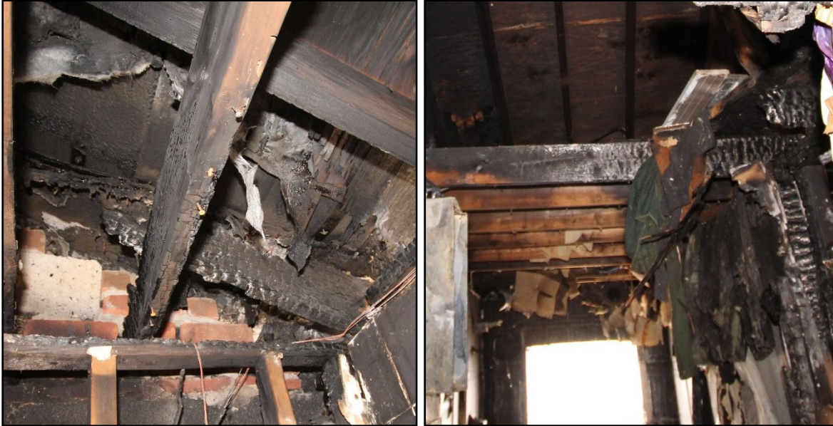
Figure 44. Lower rear section of the attic of Exposure #4 Building where the roof rafters rest on the rear wall of the second floor (left); attic space over the bathroom and hallway of the second floor of Exposure #4 Building (right).
