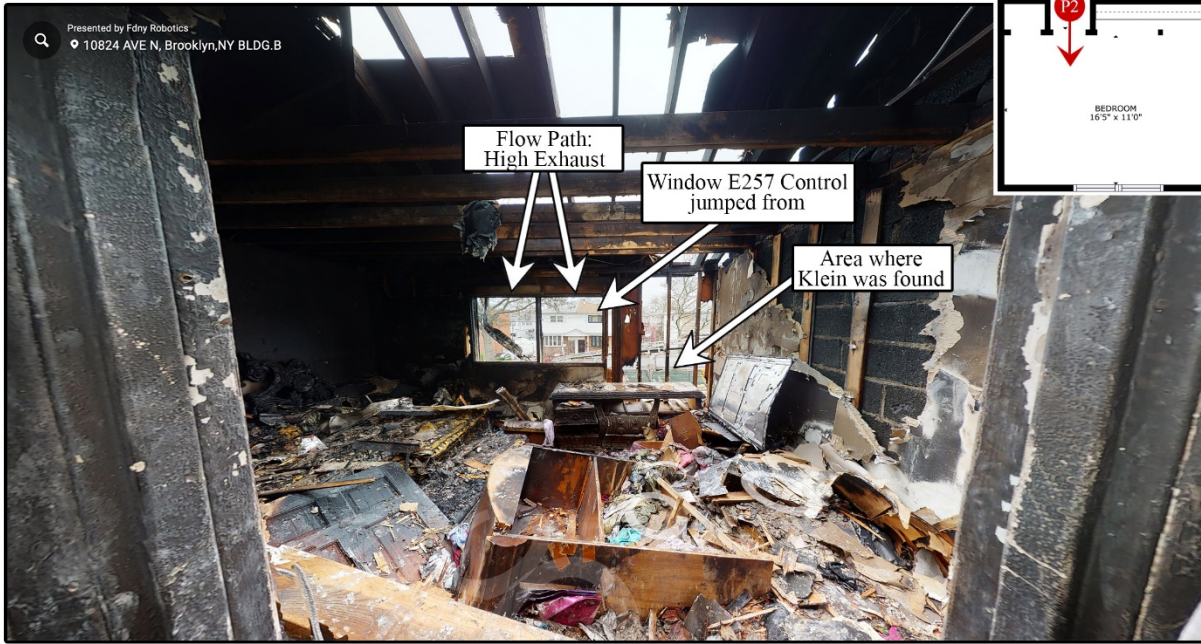
Figure 19. View of the hallway to the front bedroom on the second floor (top); view of front bedroom on the second floor, where Firefighter Timothy Klein was found (bottom).
