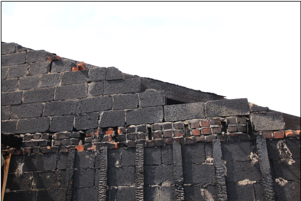
Figure 41. View of the top of the demising wall toward the front of 10826 Avenue N, where fire extended from the Fire Building to the Exposure #4 Building.
