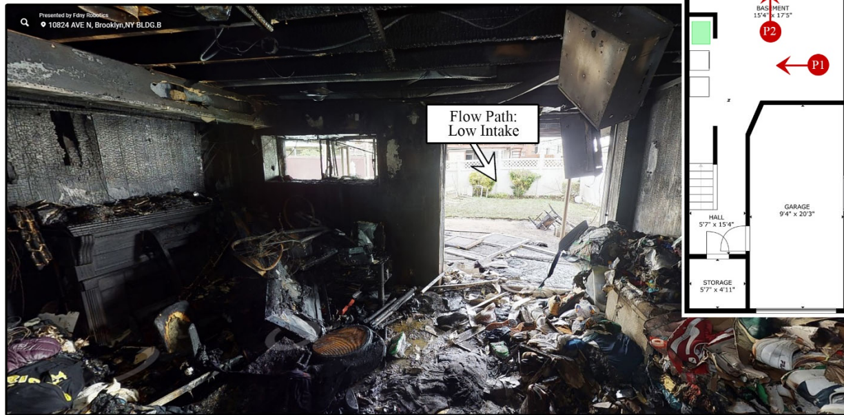
Figure 13. Photograph of utility room on the basement level of the Exposure #4 Building, showing vertical shaft and source of low intake (top); view of backyard from inside basement, showing another source of low intake (bottom).
