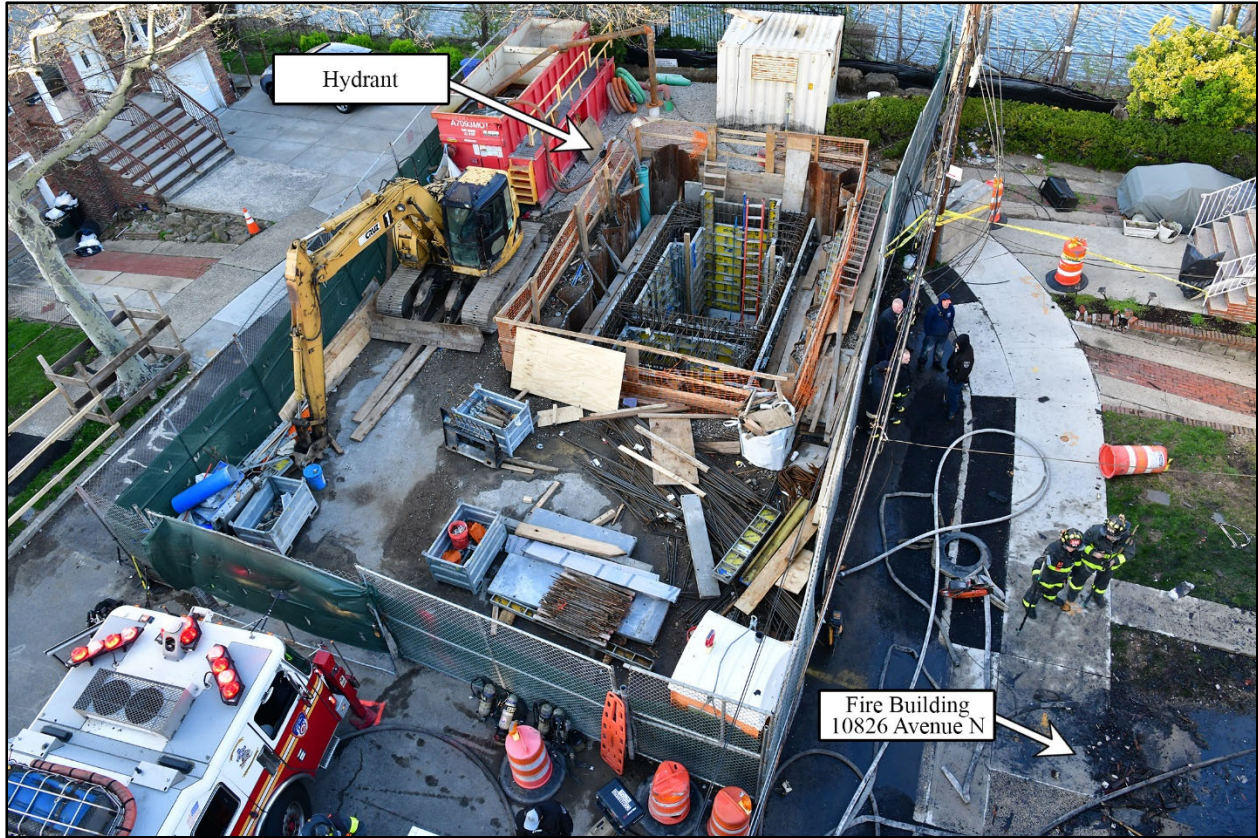
Figure 6. View of the construction zone at the dead end of Avenue N.
