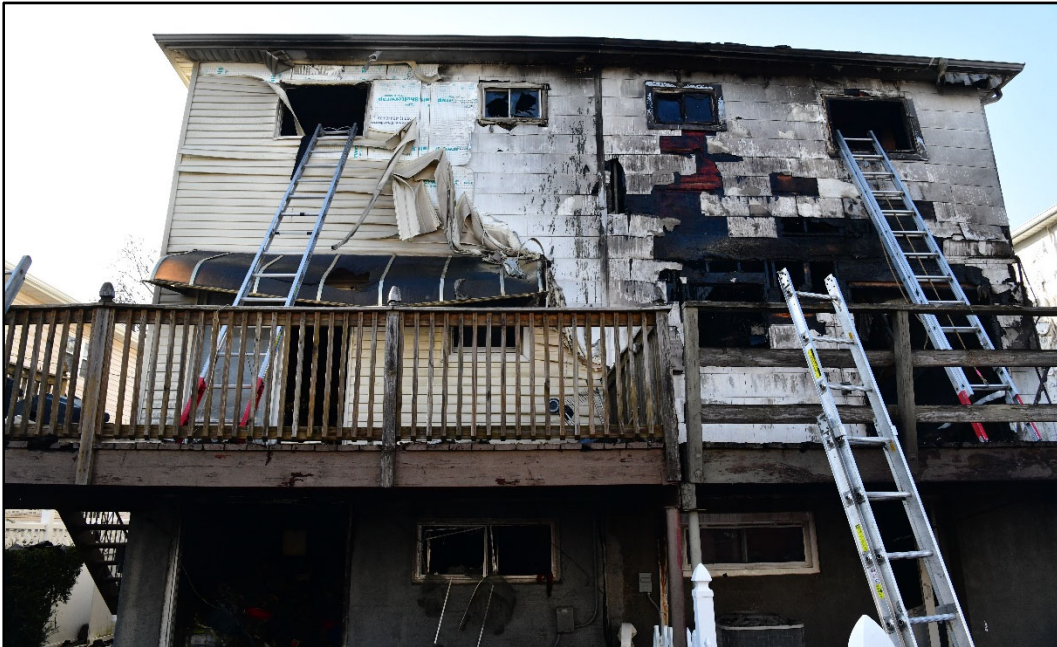
Figure 10. Aftermath of incident at rear of 10826 and 10824 Avenue N.
