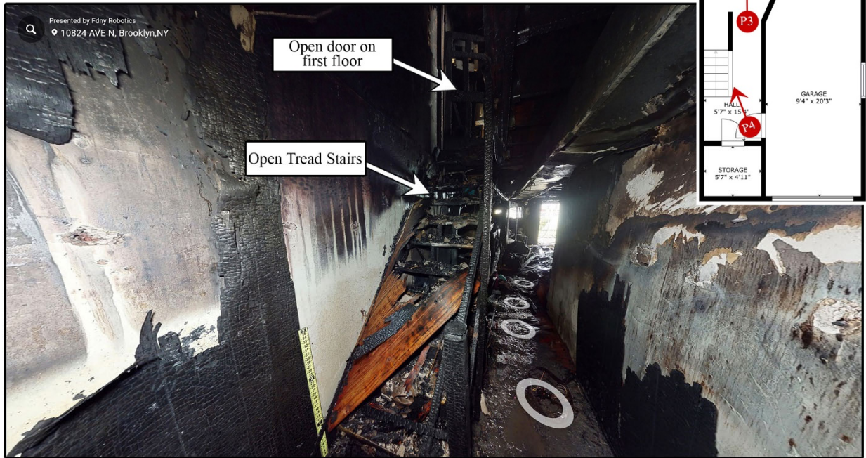
Figure 14. Basement-level hallway from front to rear, view of rear sliding glass door (top); basement-level view facing the rear of the Exposure #4 Building (bottom).
