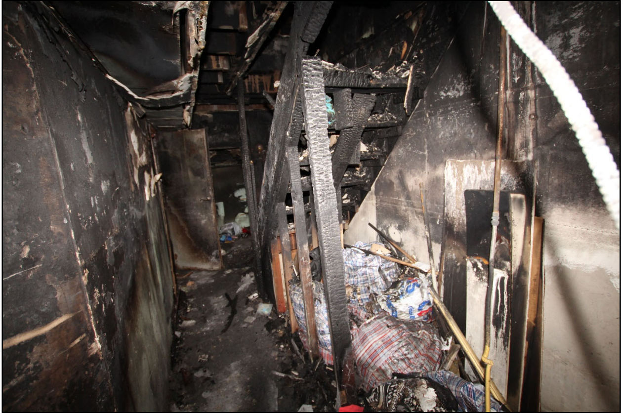
Figure 49. View from the basement level of the Exposure #4 Building from the hallway looking at the staircase to the first floor.
