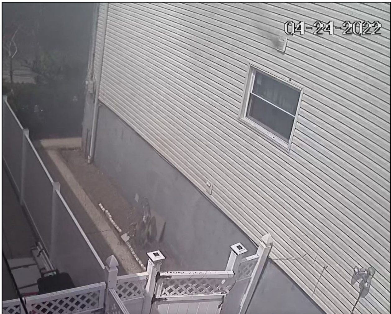
Figure 39. Side of Exposure #4 Building showing smoke from a vent pipe in the ceiling of the first floor.
