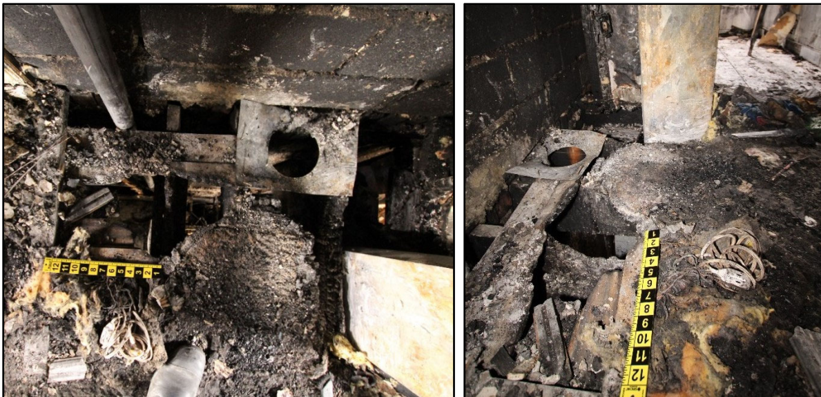
Figure 45. View of vertical shaft on the second floor looking down (left); view of vertical shaft on the second floor showing the saddle burns on the floor beams (right).
