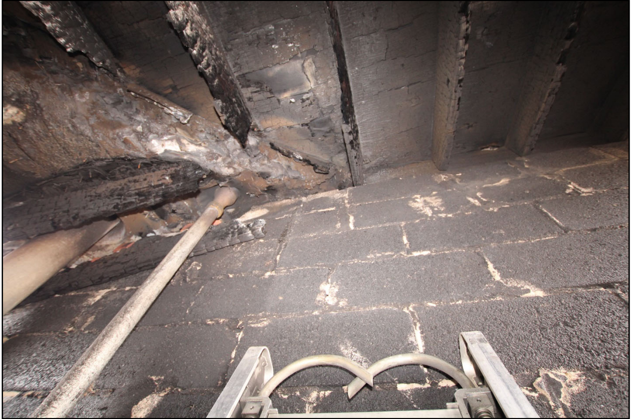
Figure 42. View of the top of the demising wall in the Fire Building toward the rear where flue pipe extends through the roofline.
