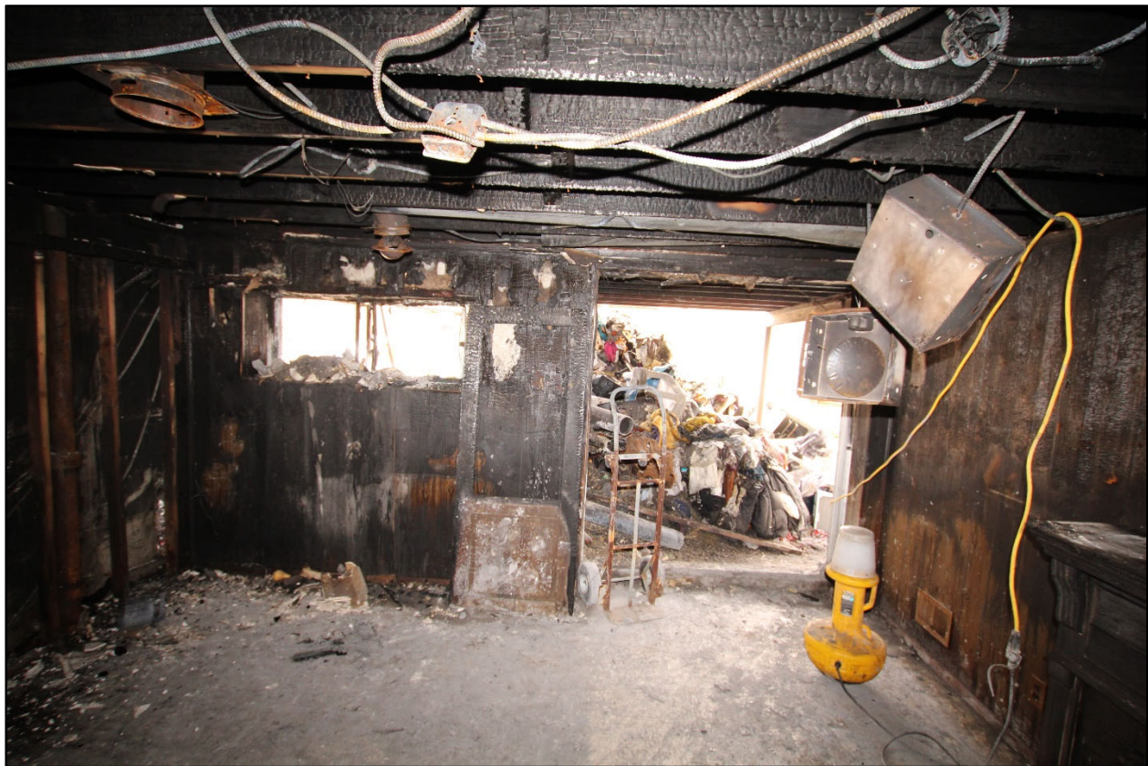
Figure 48. View of the rear exterior wall on the basement level of the Exposure #4 Building where the open sliding door provided the low intake.
