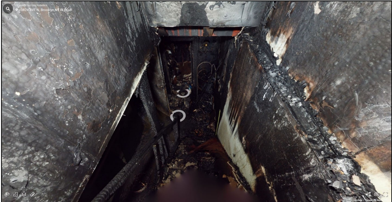
Figure 32. Burning clothes from view of the first floor into the basement of 10824 Avenue N, the Exposure #4 Building.
